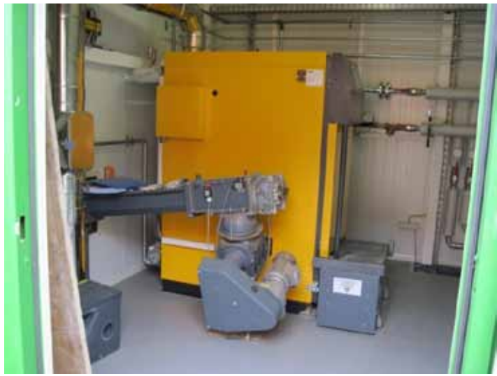
90kWth small district heating system. Photo David Coote
