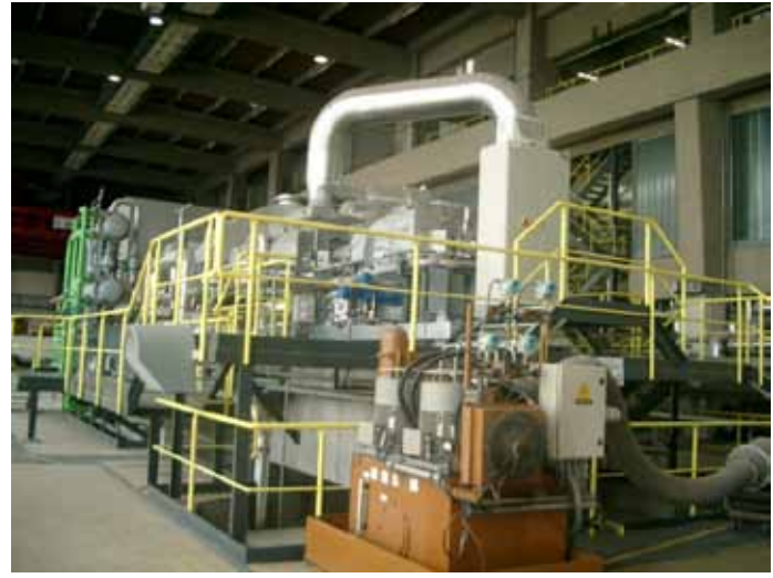
25MWe cogeneration plant turbine in Vienna. Photo Erlan Caliskan
